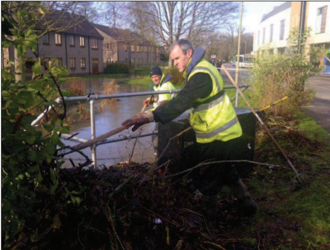
Figure 9: Environment Agency operational team removing debris from the River Bure trash screen at Hanover Gardens
