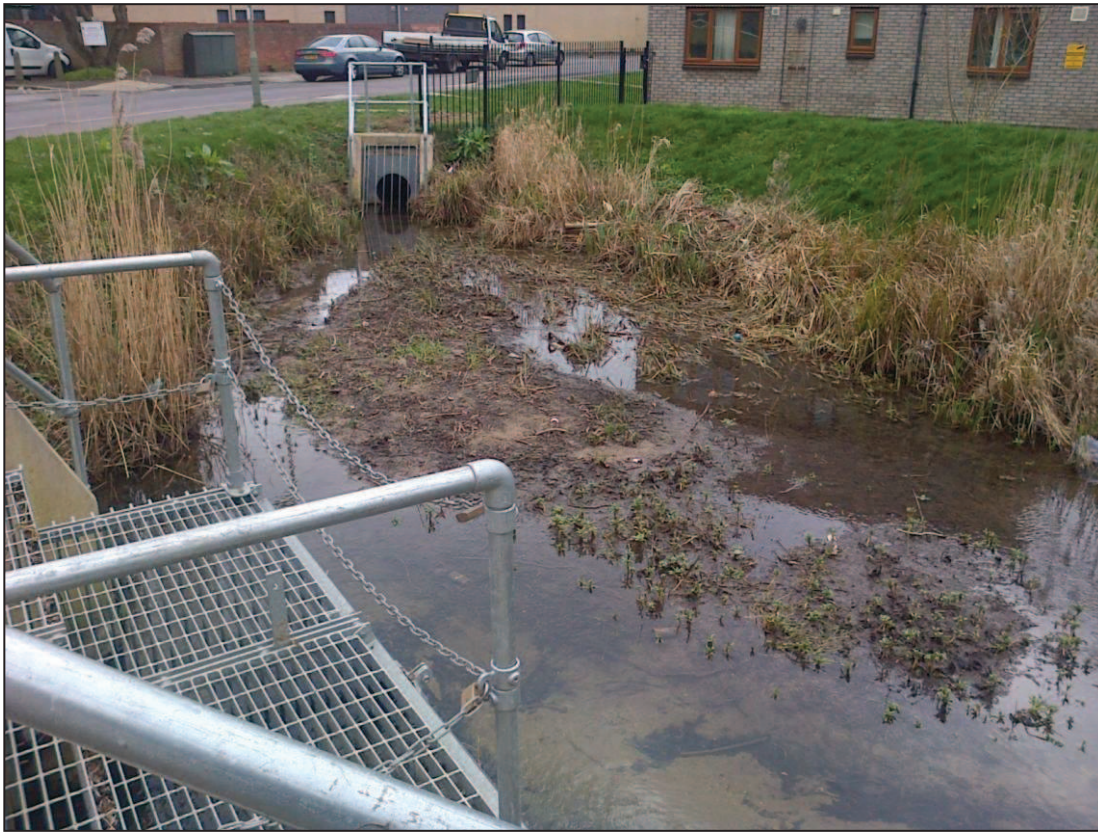
Figure 2: Trash screens at Hanover Gardens during normal flows looking south west towards the Back Brook culvert
